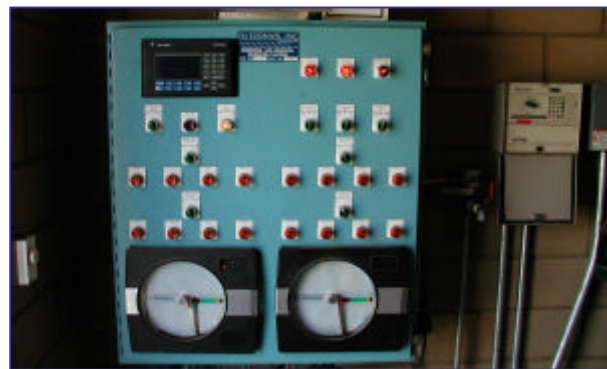
A control panel monitors operation of the new filtration unit
