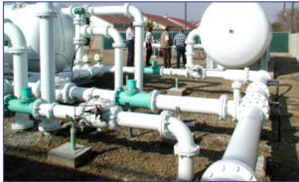
Mike Wegley, Engineer; Terry Carr, Utility Superintendent; David Weisser, Utility Supervisor and Richard Hobbs, Utility Worker, all with the City of Hanford, examine the city's new Filtronics treatment unit.
